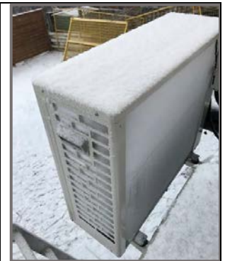
Figure 41: A Sanden CO2 heat pump water heater compressor working outside in 5°F (-15°C) weather. 89
