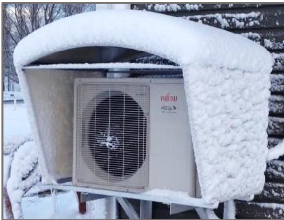
Figure 39: Fujitsu heat pump in the snow. 86
