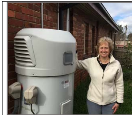
Figure 40: Jane Fisher decided to install an energy saving heat pump water heater at her investment property in Melbourne. 88
