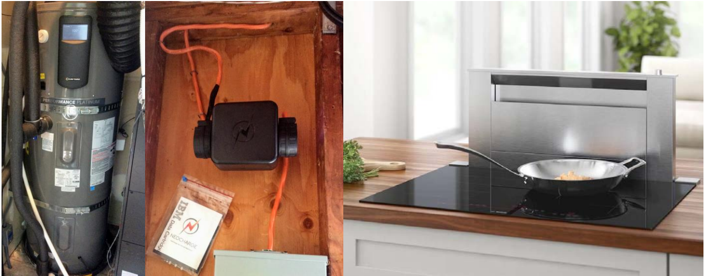
Figure 26: At the Schmidt’s home, the Bosch electric induction stovetop 68 is shared on the same circuit as the Rheem heat pump water heater 69 using the NeoCharge (middle) (Images courtesy of Steve and Lisa Schmidt).
