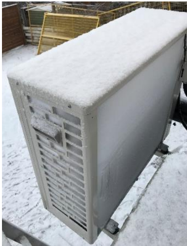
Figure 42: The Eco2 heat pump water heater compressor working outside in 5°F (-15°C) weather. 91
